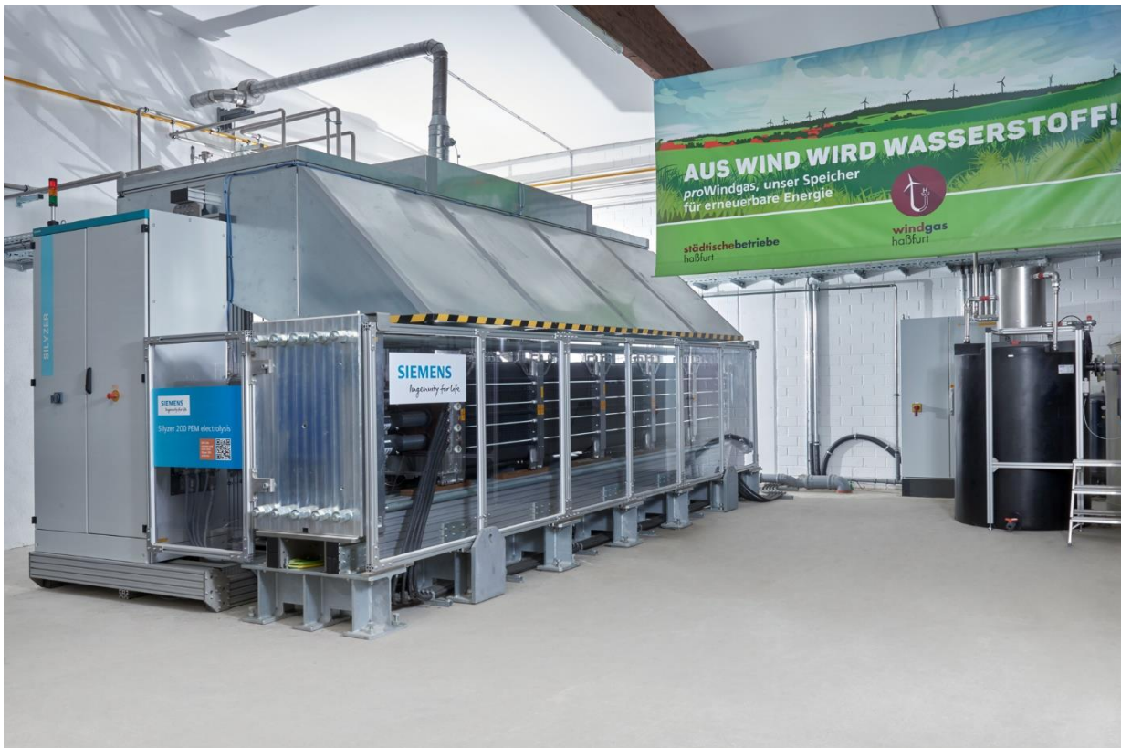
The Silyzer 200 (1.25 MW output) electrolyser from Siemens at the Stadtwerk Haßfurt is used to produce hydrogen with excess electricity from renewable energy generation plants. Image source: Stadtwerk Haßfurt GmbH
