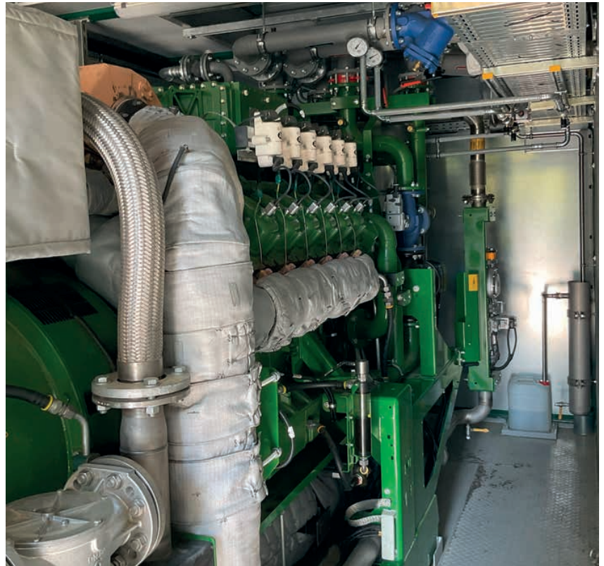
Figure 1. Avus 500plus from 2G Energy in use at Lorenz
