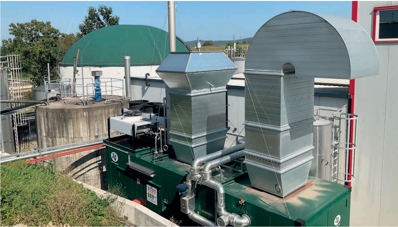
A biogas facility and a CHP system are part of the sophisticated energy concept for the production of snacks
