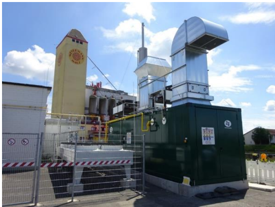
Figure 1 In Haßfurt, green hydrogen is produced locally and converted back into electricity
