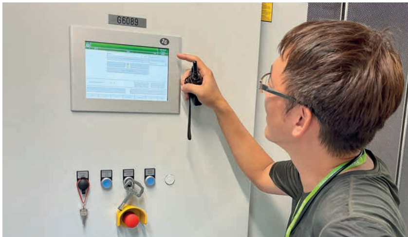
Figure 2. The well-established 2G control system allows a continuous and reliable hydrogen CHP operation
