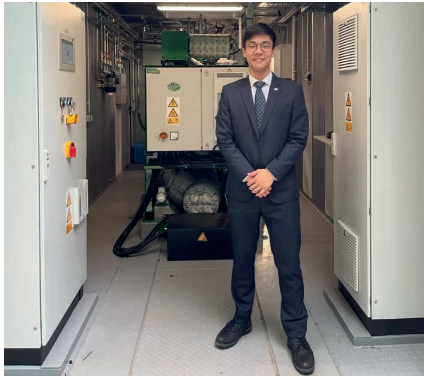
Figure 1. Andrew Lee of AM-Power has managed the installation of the project on site
