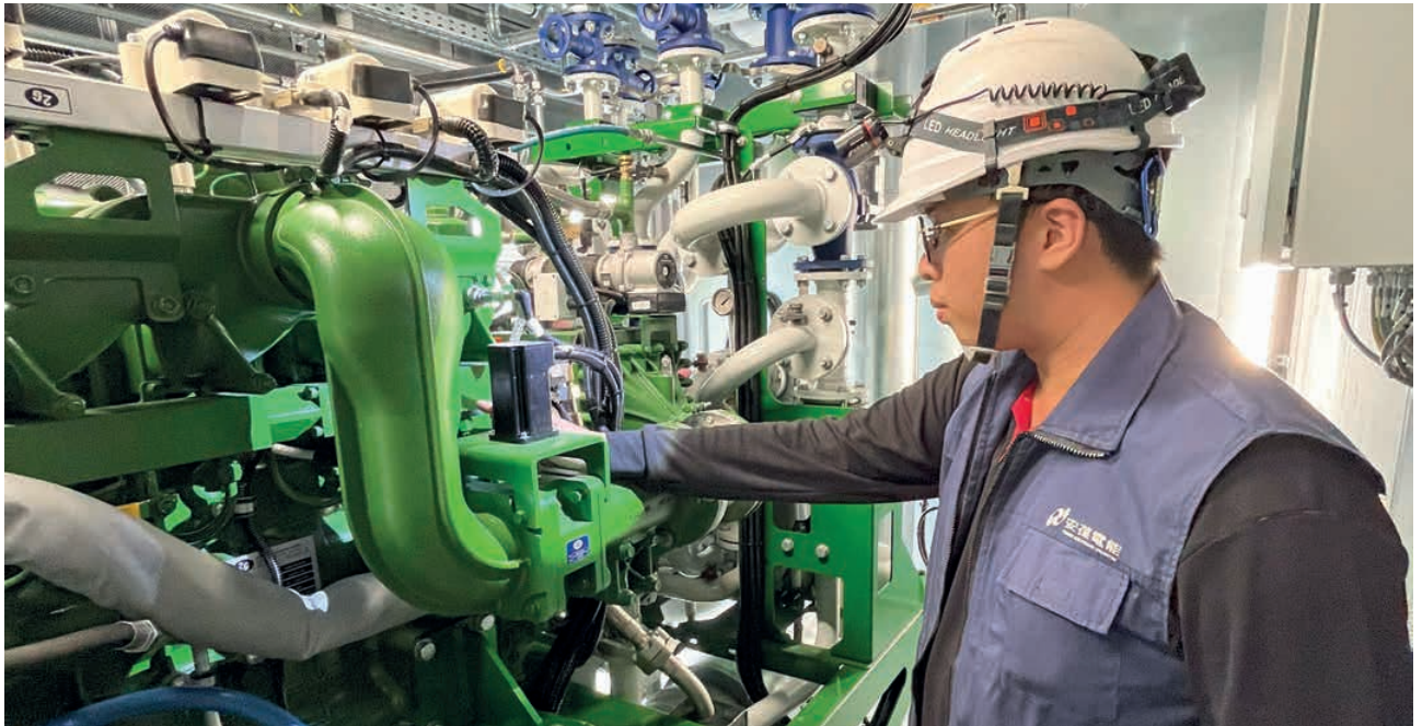
Hydrogen, which is a by-product of a recycling process, is used in this engine to efficiently generate electricity and heat
