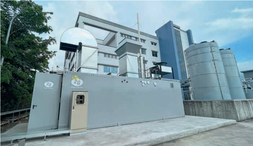
Figure 3. Both the engine and the hydraulics as well as the complete control unit were delivered in a tailor-made container
