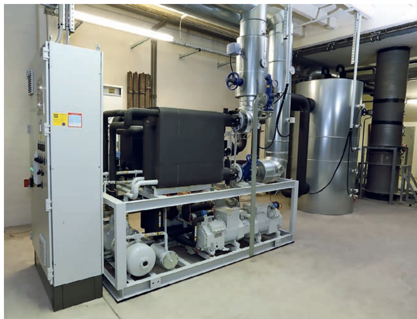
Figure 2. Heat pump which is integrated into the CHP project in Bad Lauterberg
