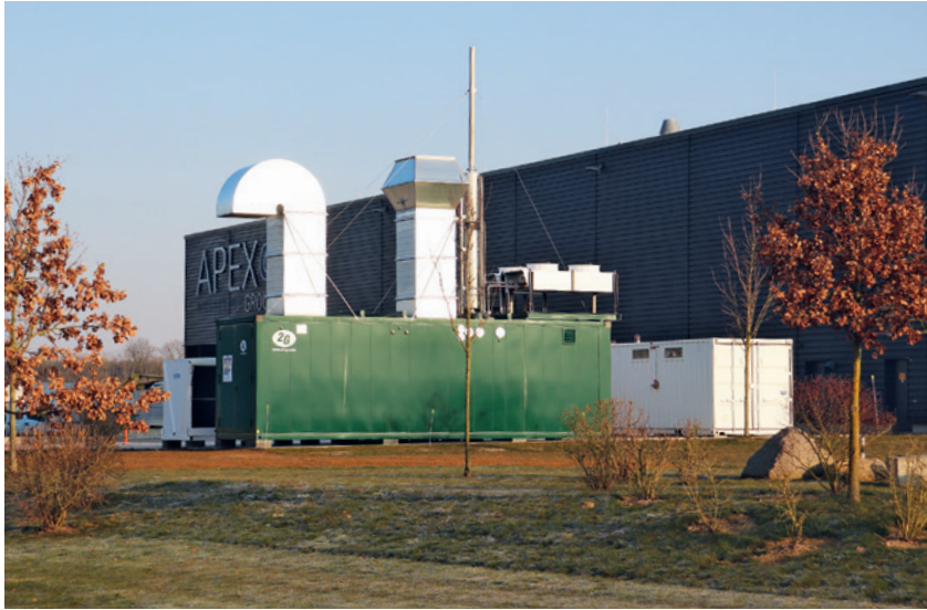
Figure 4. The CHP unit in Rostock/Germany is operated with 100% hydrogen
