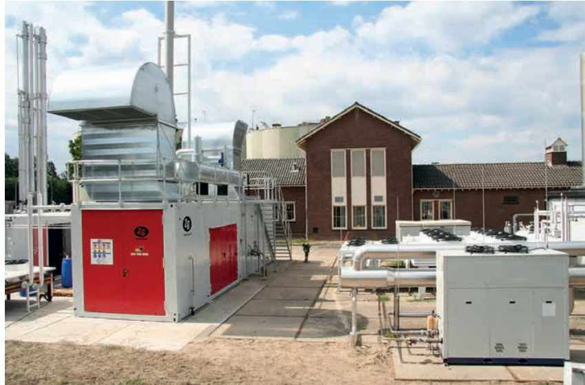
Figure 1. CHP improve both energy self-sufficiency and environmental performance of treatment plants
